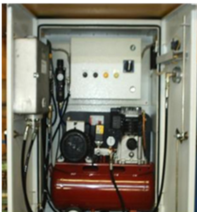
Compressor with Control
