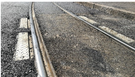
Flange and railhead lubrication
